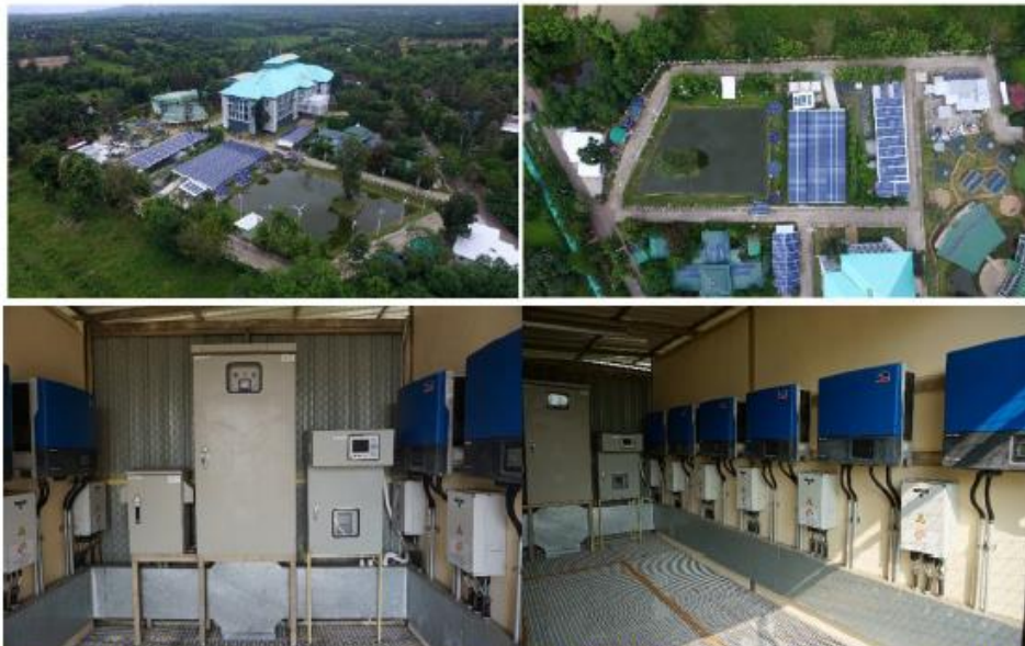
Project 1: Rooftop photovoltaic power plant capacity 300 kWp. (operating date: November 2017)
