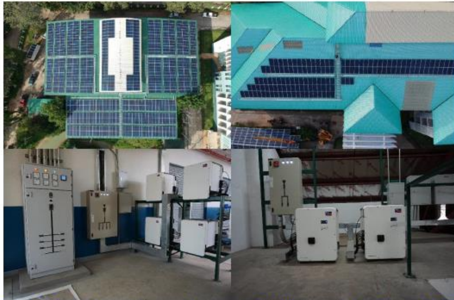
Project 2: Rooftop photovoltaic power plant capacity 300 kWp, (operating date: December 2020)
